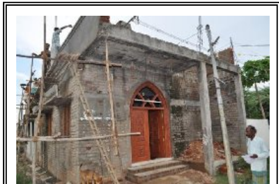
St. Thomas Lutheran Church, Kannigapuram, Pastor: Rev. LSD. Gladson Premkumar. Members 180, Communicant Members 50. Area of Construction : 1584 Sq.Ft. Requirement: INR 150,000 (about $3300)
